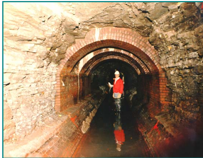
Some of the old brick arch work (Norton Street) in Rochester's combined sewer system.
