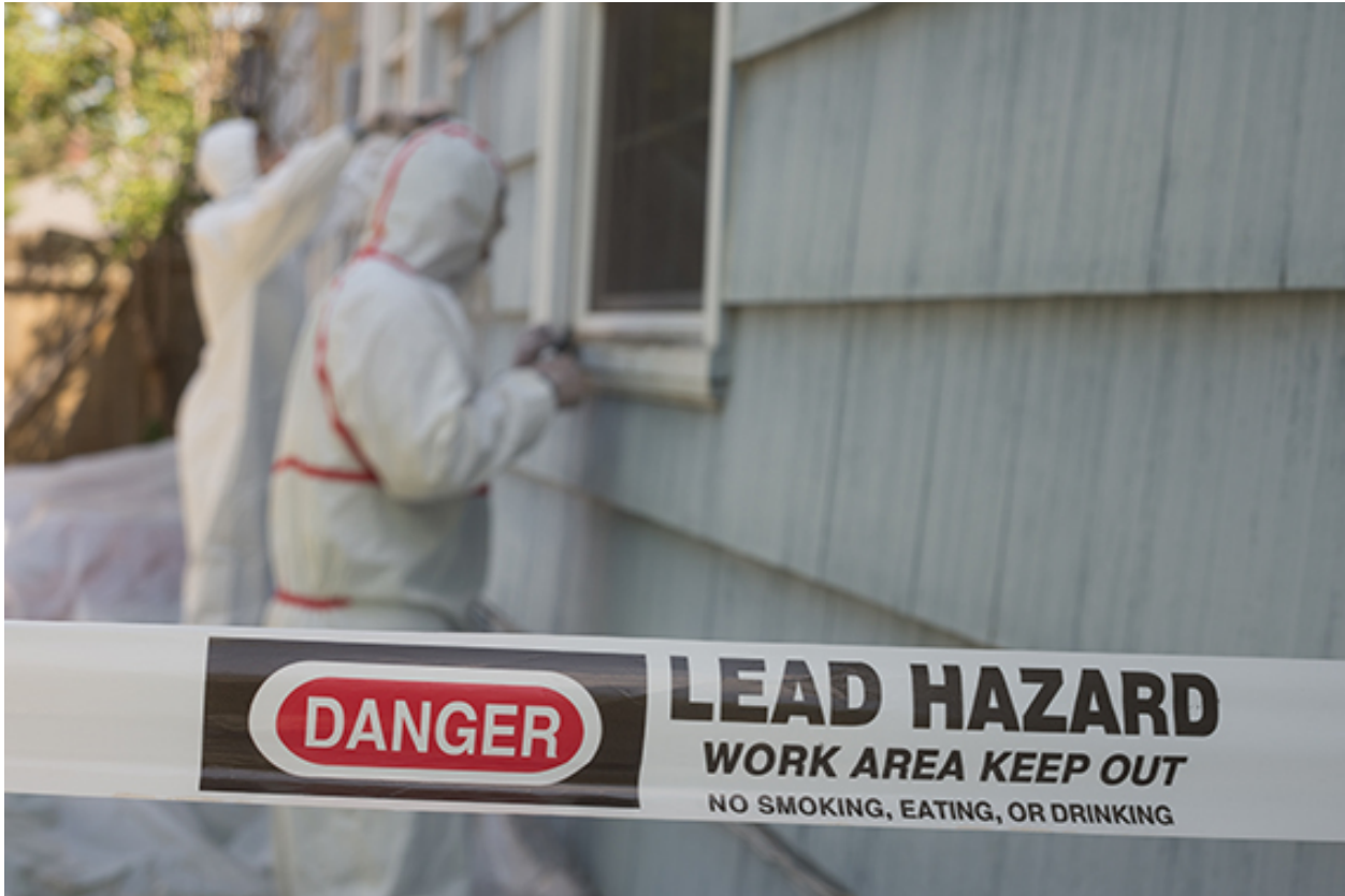
Lead Paint Cover Photo
